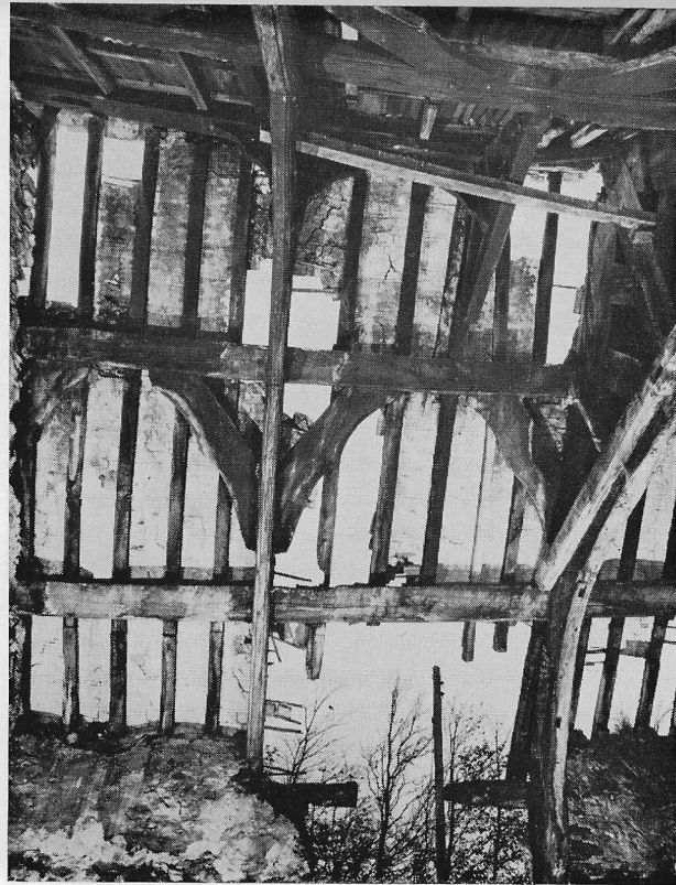
FIG. 11. View of North bay B-1, 1-C showing lower. Note windbrace survivors showing former existence of truss B
