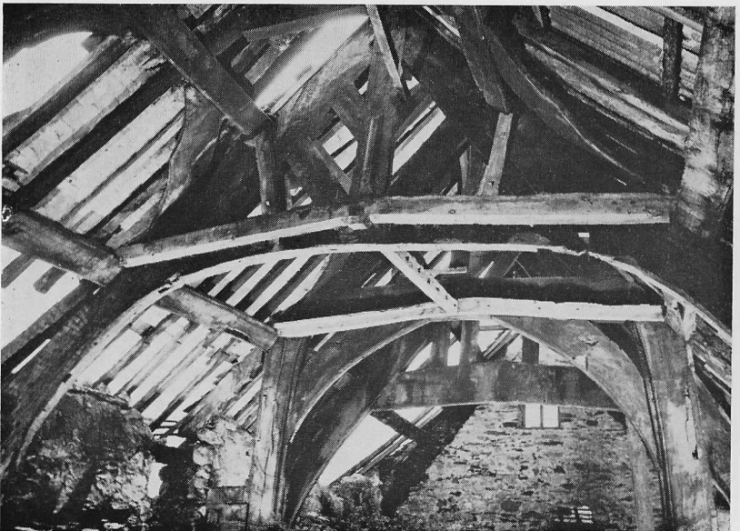
FIG. 13. General view showing louver truss, truss G, truss 2, and trusses D and E
